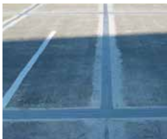
Joints de dilatation
